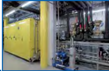
Air conditioning and exhaust air technology
